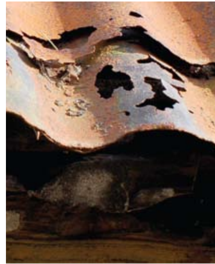
Accelerated corrosion by overlaying sheets and causing capillary action
