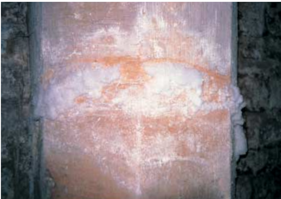
Figure 21 Masonry suffering the effects of damp: a 'cushion' of efflorescing salts has developed around a joint in this sandstone pier as the saturated masonry has dried out. (John D. Stewart)
