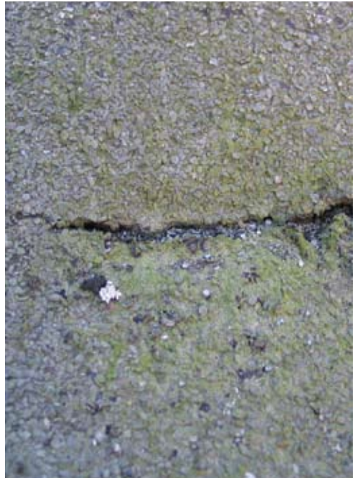
Tear in roof felt
