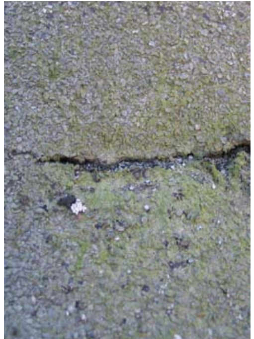
Tear in roof felt
