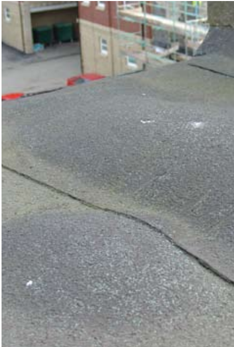
Blistering of roof felt
