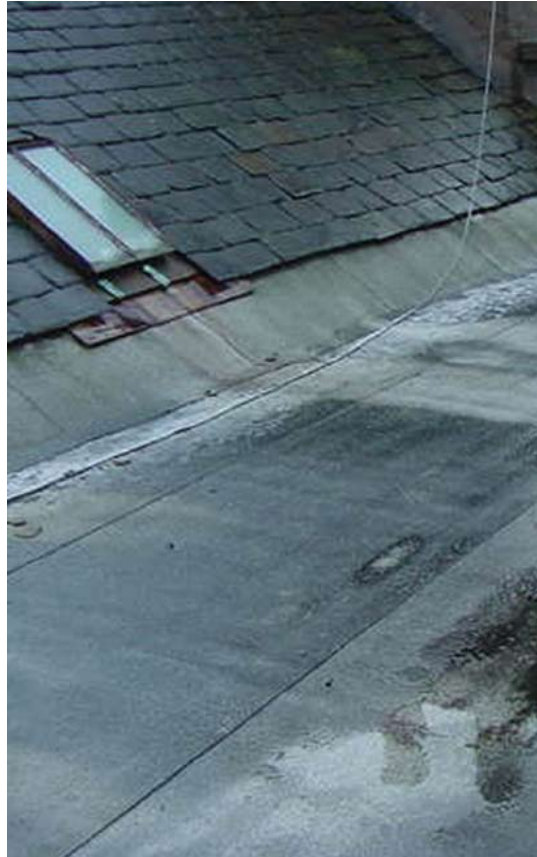
Standing water is a major source of deterioration in flat roofs
