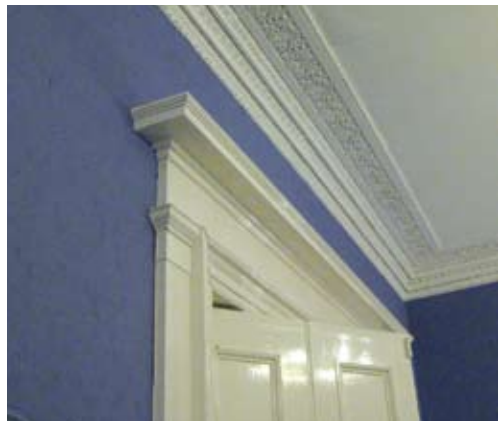
Hidden ventilation features in Randolph Crescent, Edinburgh – The pediment above the door admitted warmed air, and gaps in the cornice (now blocked) allowed it to be drawn away.
