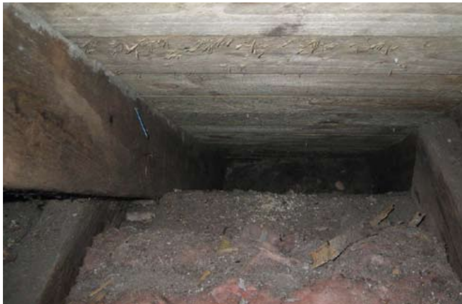
Fig 5. Loft insulation fitted, but the coombes are kept clear for air movement.
