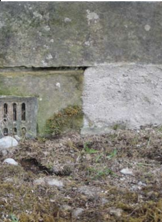
Grate blocked; note also the risen ground level.
