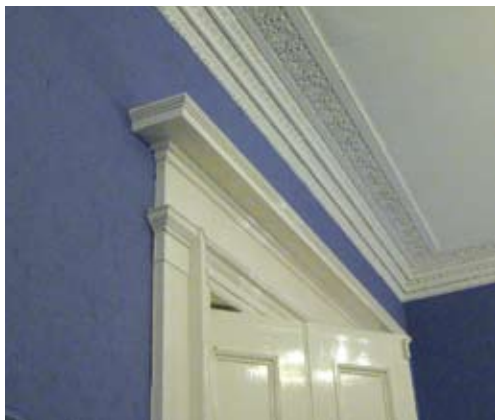
Hidden ventilation features in Randolph Crescent, Edinburgh – The pediment above the door admitted warmed air, and gaps in the cornice (now blocked) allowed it to be drawn away.
