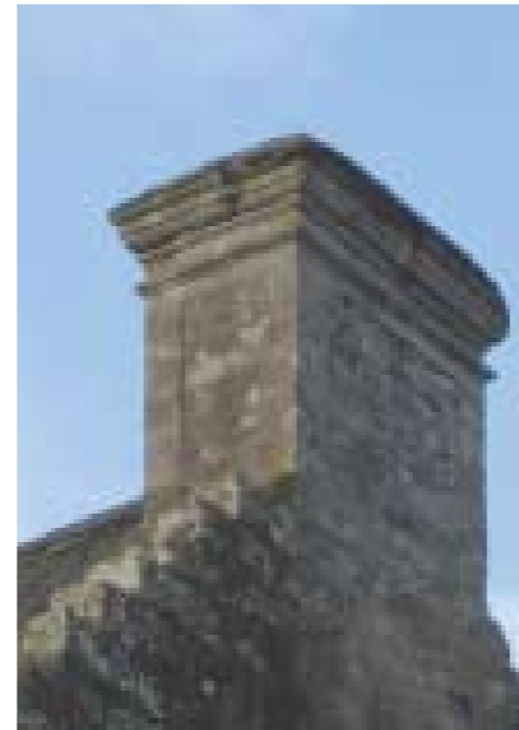
Banding on this late 17th C chimney.
