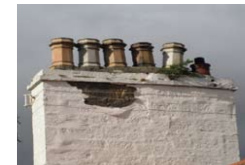
A mid 19th C chimney and cans showing a variety of problems.
