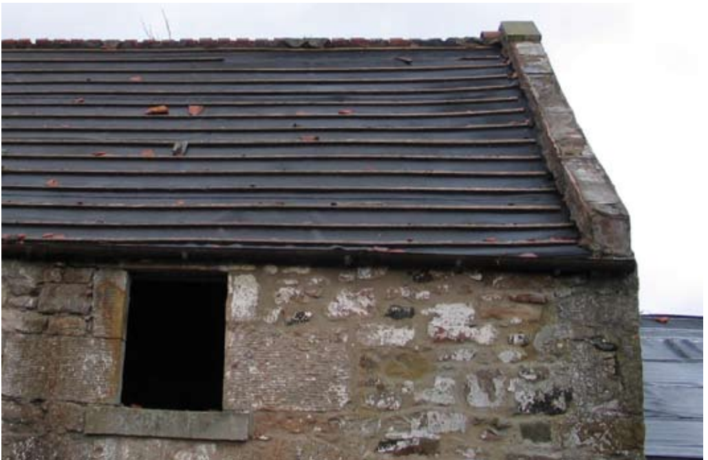
An exposed roof showing battens onto which pantiles are hung by their nibs
